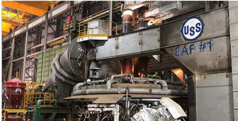
Electric arc furnaces, like this one in Alabama, will be used at U.S. Steel's new facility in Mississippi County.
